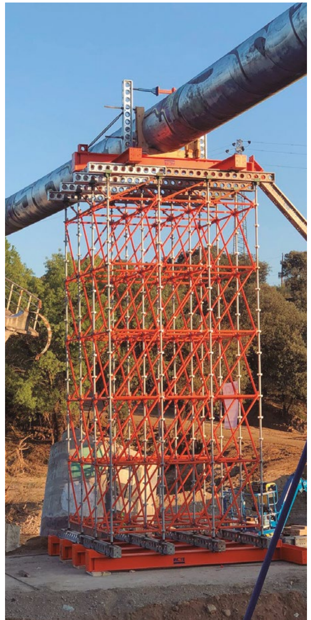
Bridge that supported the main supply pipeline of Picadas, Toledo, Spain, affected by DANA.
