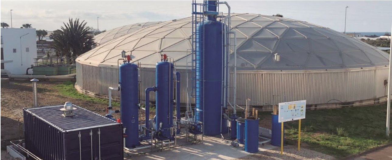
Life Ulises project located at the El Bobar WWTP, Almería, Spain.
