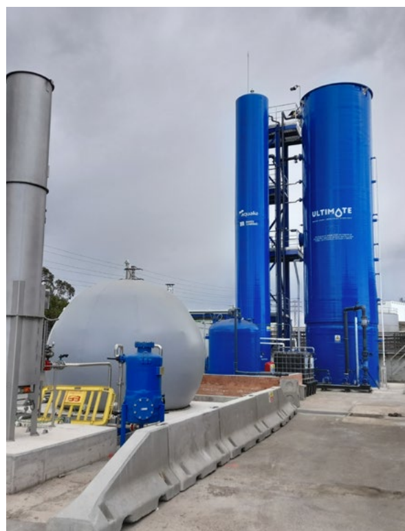
Project installed in the Mahou-San Miguel company, Lleida, Spain.
