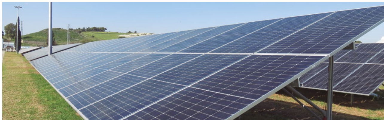
Solar panels installed at the WWTP in Jerez de la Frontera, Cadiz, Spain.
