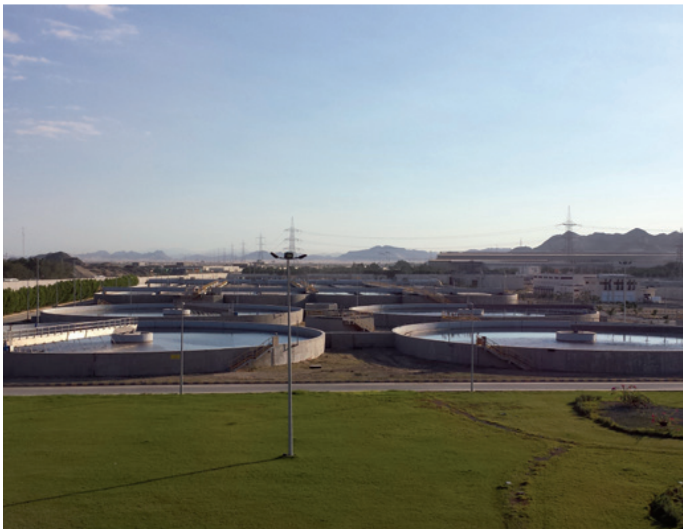
Wastewater treatment plant in Mecca.
