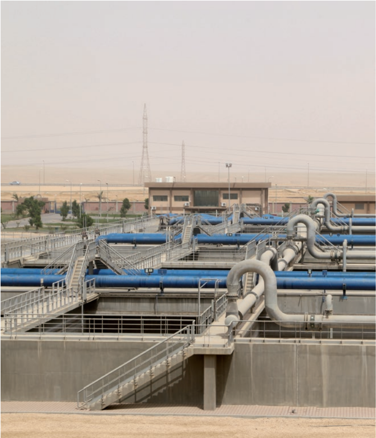
New Cairo WWTP.
