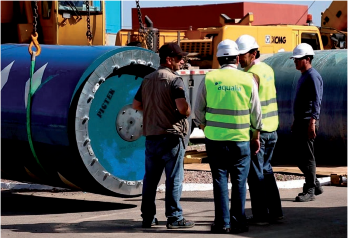
PIG technology applied for cleaning water intake pipes in the Mostaganem, Algeria, desalination plant.
